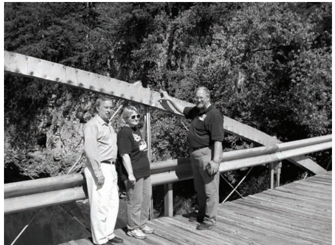
IHPA Executive Director Mike Kramme, Board Member Rosemary Rohr and bridge inspector Dennis Waugh during the inspection of the Hale Bridge
