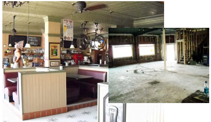
Progress being made at 1127 3rd St SE in Cedar Rapids. IHPA assisted the owners in accessing state and federal tax credits and a historic property tax exemption.
